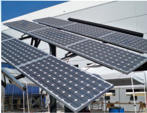
Solar array for mid-sized water purifier.
